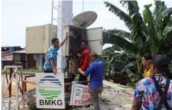
Figure 4. Reactivation of Jayapura City Tsunami Early Warning Siren Source: BMKG Region V Jayapura, 2024
