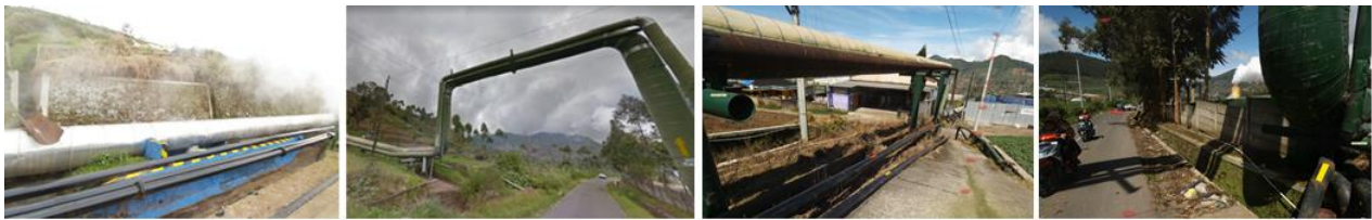
Figure 2. Pipeline network: (a) an open area with a shiny metallic colour; (b) a curved vertical pipeline at a road intersection with matte colour; (c) the steam pipe is above ground supported by its support and the water pipe is below the steam pipe; (d) segments of the steam pipe and water pipe are covered by vegetation so that they cannot be seen from above.
