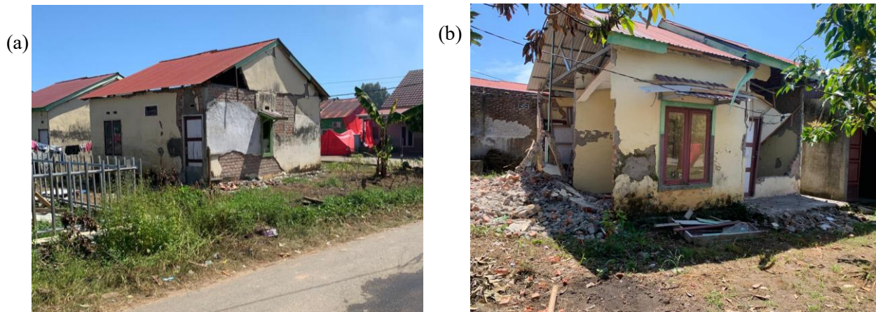
Figure 1. (a) Damage to building walls caused by the May 23, 2025 earthquake in the Rafflesia Asri Housing Complex (b) Damage to structural elements of buildings at the research site.
