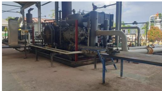
Figure 1. KN – 02 Gas Compressor
