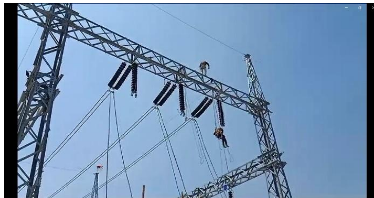
Figure 6. Work Failing to Attach a Full Body Harness to the Anchor Point While Working at Height
