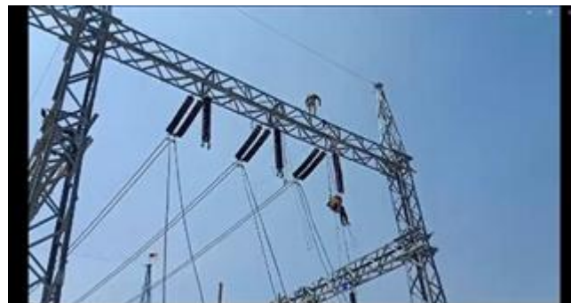
Figure. 3. Work Failing to Attach a Full Body Harness to the Anchor Point While Working at Height
