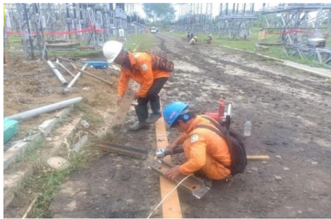
Figure 5. Worker Smoking and Operating a Grinder without a Safety Cover
