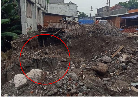
Figure 3 Identification of strauss pile failure
