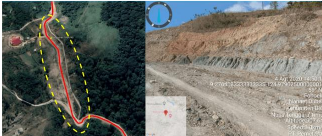
Figure 1. Current Motaain-Henes-Motamasin Road STA.149+140 Landslides Source: East Nusa Tenggara Province P2JN, 2020
