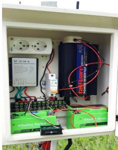
Gambar 12 Panel box and electrical components.
