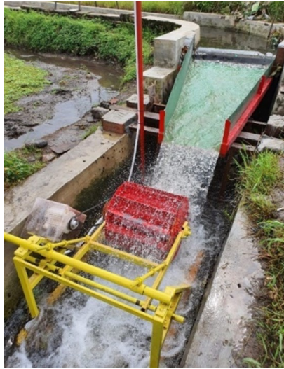
Gambar 11 Crossflow turbine instalation.
