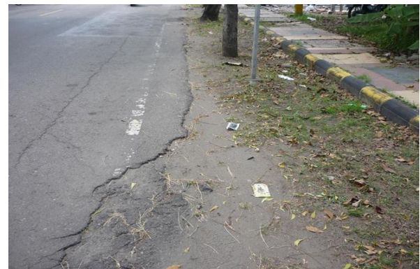
Figure 2 Shoulder of D.I. Panjaitan Road, Madiun City KM 1 + 100.
