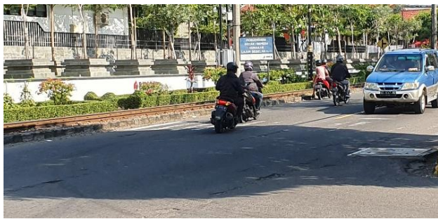
Figure 4 Road Construction Strength on Yos Sudarso Road KM 1 + 900.
