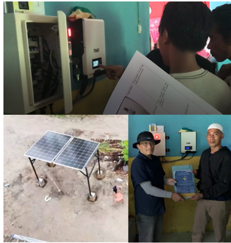
Gambar 6 Hasil akhir instalasi sistem BIM-Fish di plant-site .
