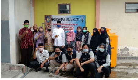
Gambar 7. Instalasi filter air di SMPN 1 Karanggeneng Lamongan
